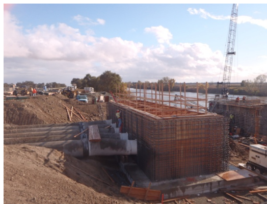
Discharge pipes and valve vault walls
